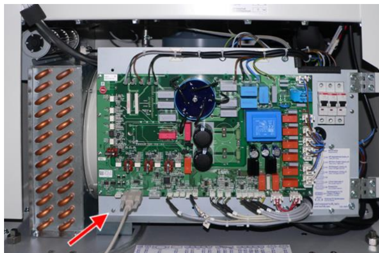
Fig. 10: Position of the screw for loosening the power module
